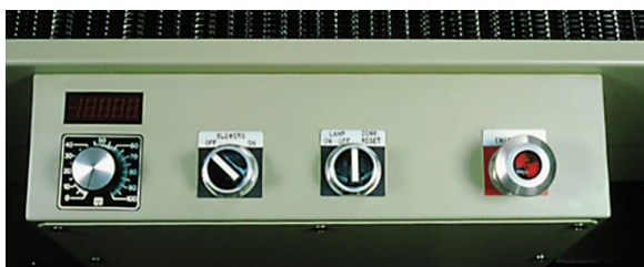
System control panel
