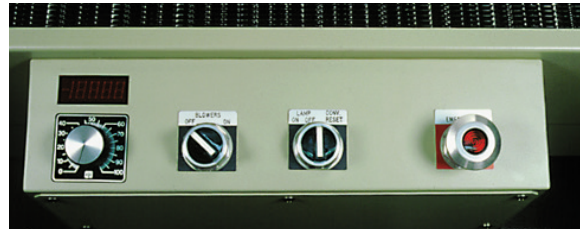
System control panel.
